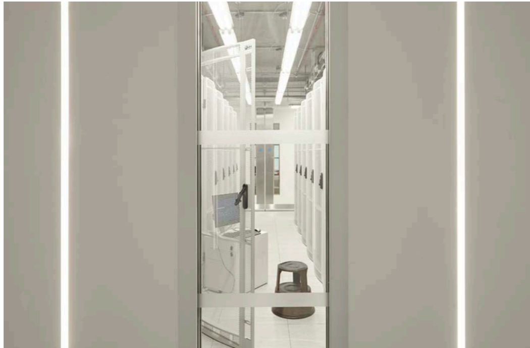
12 Glimpse of the main equipment room with servers. The BDI processes and stores significant amounts of data on a daily basis, with its server room providing enough computing power for 600 trillion computations per second.
