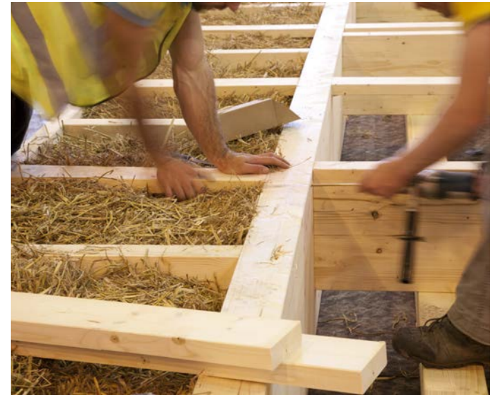
5 Straw panels constructed on site. Our environmentally friendly design was informed by Sutton Bonington's strong agricultural heritage and sustainability track record.
