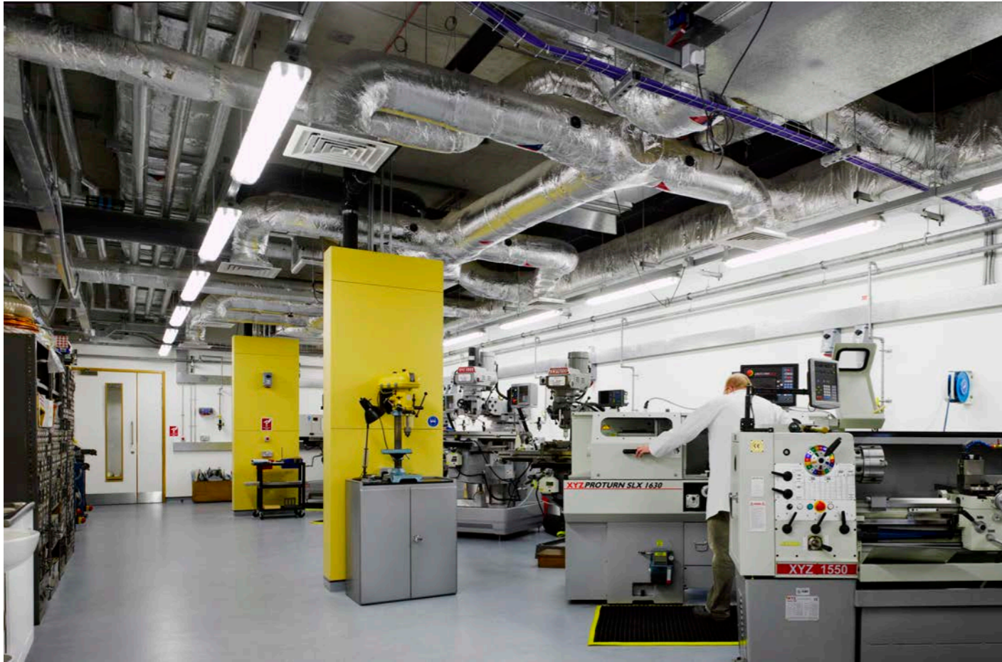
14 Lab spaces in use. The building's highly efficient plant reduces the energy consumption of this high-tech research building.
