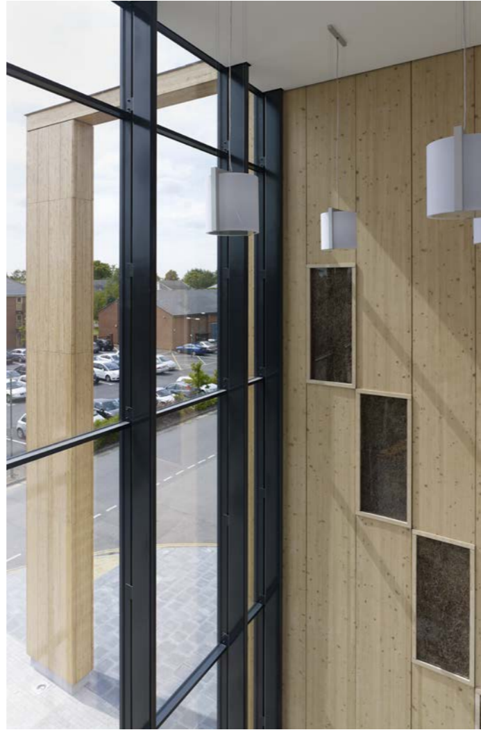
12 View of the exposed straw via truth windows that reveal it to passers-by.
